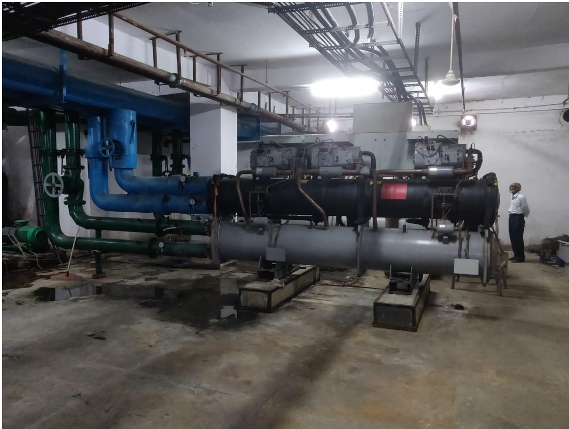
Fig. Chiller system at KGMU
