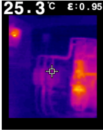
DESCRIPTION –CHILLER-4 Main panel surface temp-25.3
