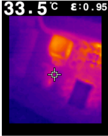
DESCRIPTION CONDENSER PUMP-1 Panel surface temp-33.5
